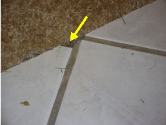
End broken off of entry area floor tile
