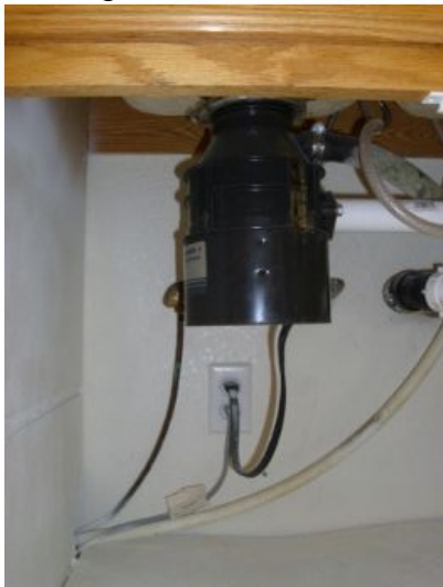
Garage disposal jammed
