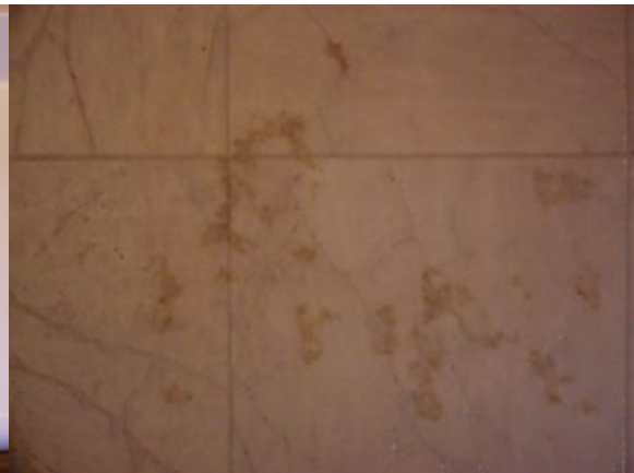
Stain on vinyl flooring in bath - cosmetic
