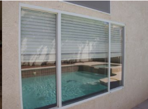
Missing solar screen
