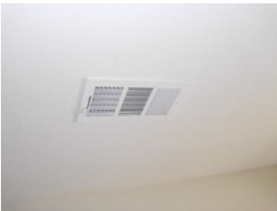
Air condition register
