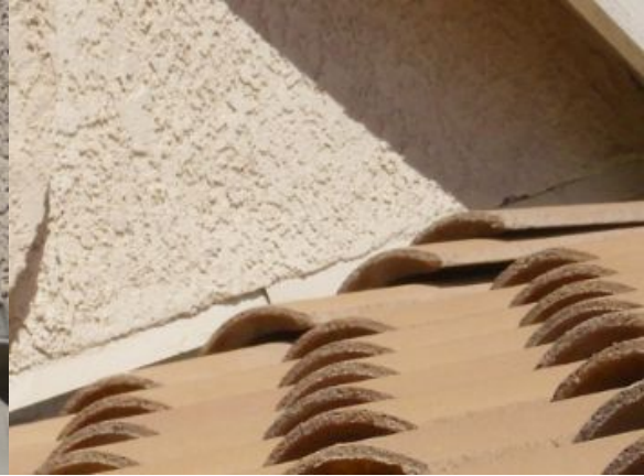
Loose tile on roof
