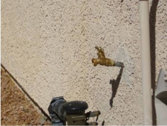
Front and back faucet missing backflow diverter
