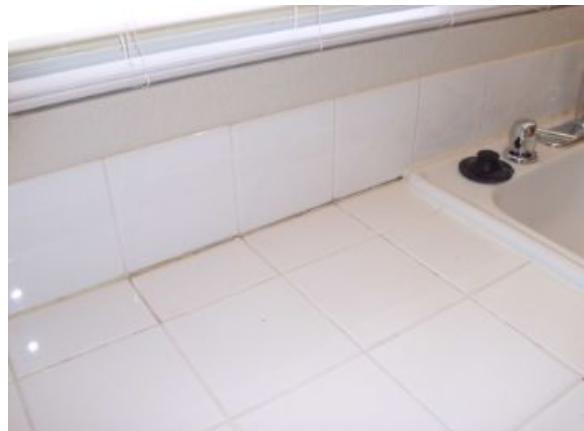
Crack in grout line
