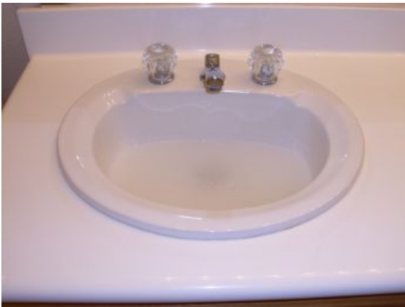
Slow drainage in all bathroom sinks
