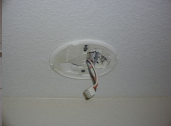
Missing smoke detector
