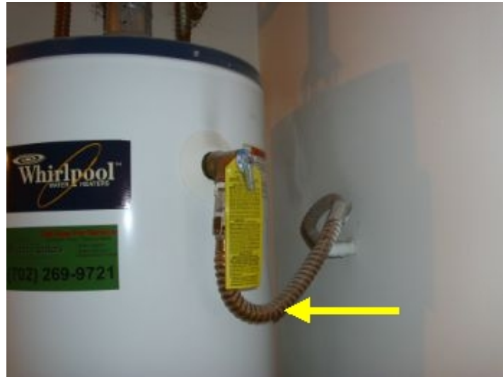
TPR valve should not have water trap
